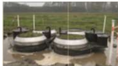
Lysimeter stations after the installation of the waterproof collars and dismantling of the groundwater lowering
