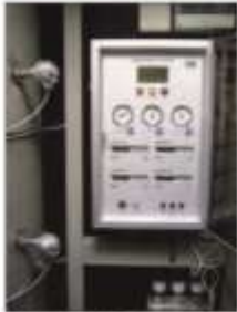
Fully automated by the control unit
