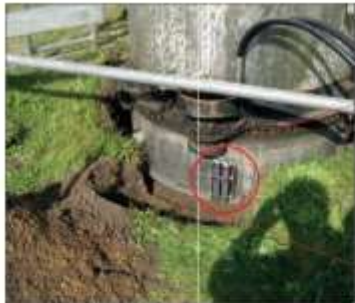
A wireless camera watches the cutting process to accomplish a well controlled cutting process
