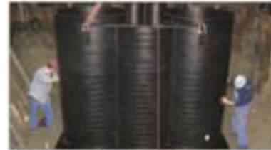
Utilization of the excavation pit for the installation of two 2-tile container lysimeter stations
